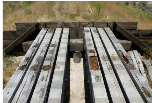
Figure 22: Trestle #2 stringers showing pockets of deterioration on the top faces.
