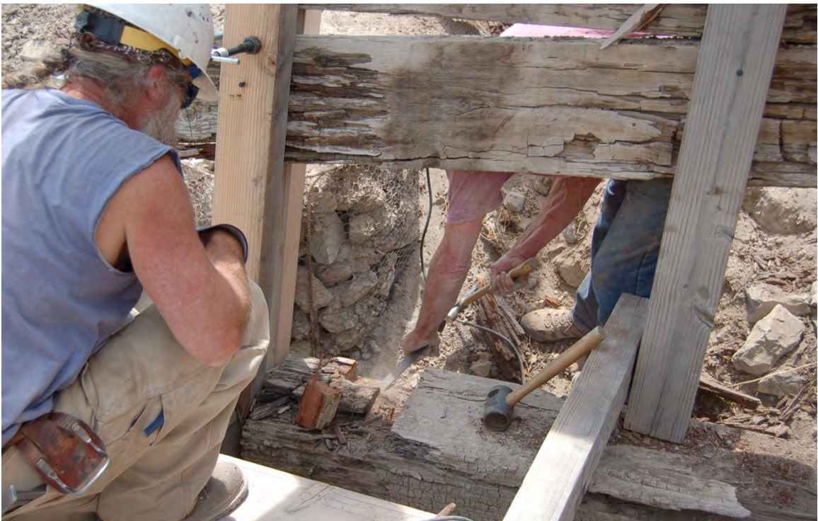
Figure 64: A section of the intermediary sill at the west bent was found to be soft as the result of decay. The section was removed with a reciprocating saw and later filled with an in-kind replacement block.
