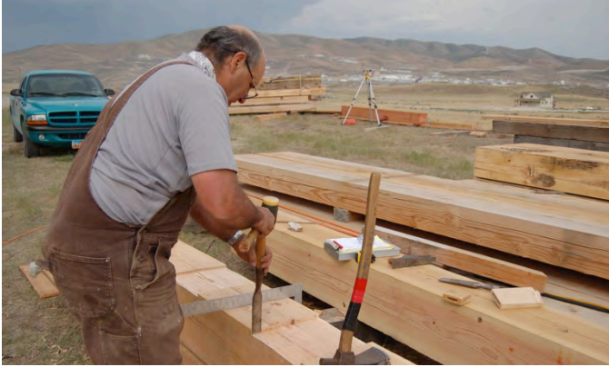
Figure 30: Squaring a mortise in a replacement pile cap with a chisel. The joints are laid out to fit the tops of the piles.
