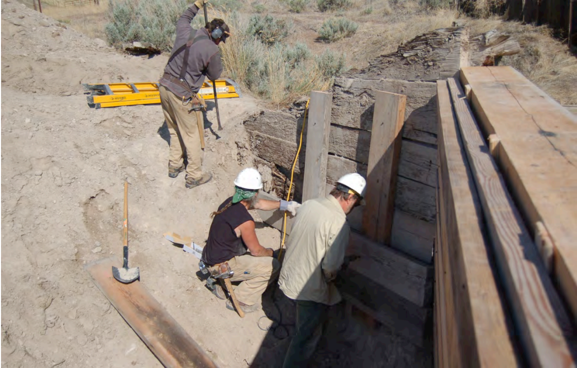
Figure 69: A second layer of planking was also applied to the back of the northwest wing wall to provide additional stability for the remaining original members.
