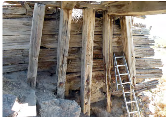
Figure 14: East bent piles with severe deterioration.
