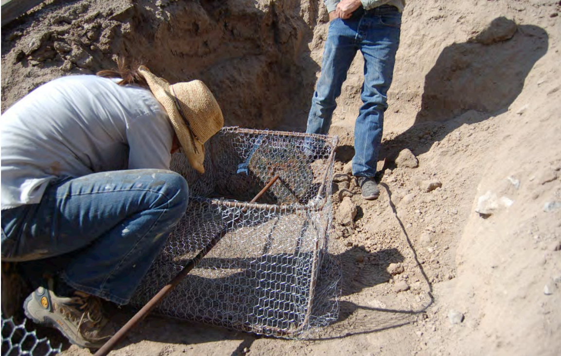
Figure 73: A deadman was installed behind the west bulkhead to add stability and to help prevent further twisting of the west bent.
