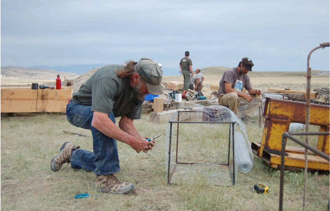
Figure 72: Replacement gabions were welded from #4 rebar and covered with two layers of wire netting.
