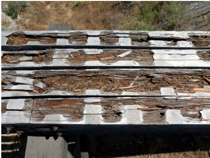
Figure 36: Extensive decay was found along the stringers of Trestle #2.
