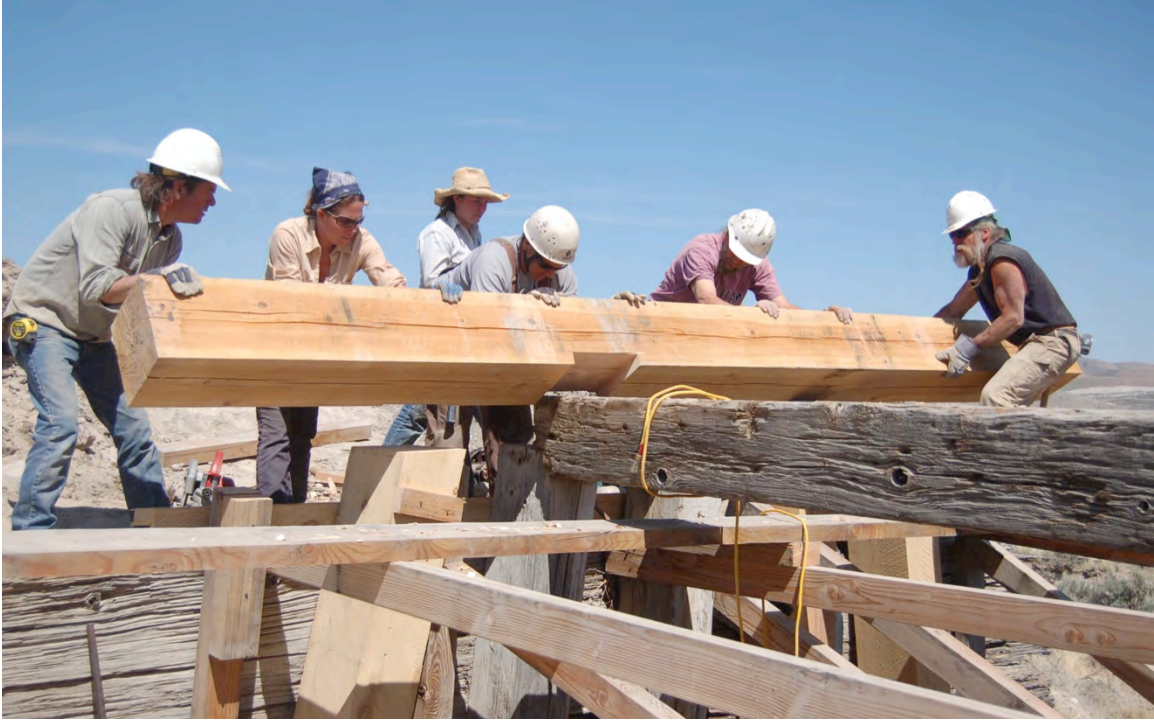
Figure 79: Replacement timbers were extremely heavy, often weighing several hundred pounds, and took several people to move them safely.
