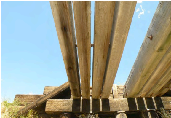
Figure 23: Trestle 2 stringers appeared sound when viewed from below, but all had internal deterioration.
