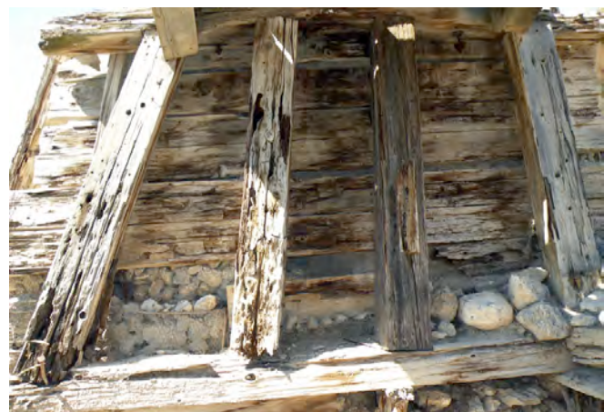
Figure 15: West bent piles with visible deterioration.
