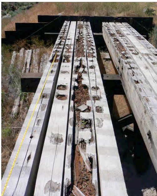
Figure 3: The stringers of Trestle #2 had extensive decay pockets along their length.
