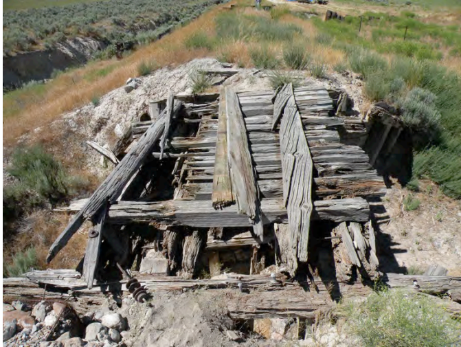
Figure 2: Many of the members of Trestle #1 were badly deteriorated.
