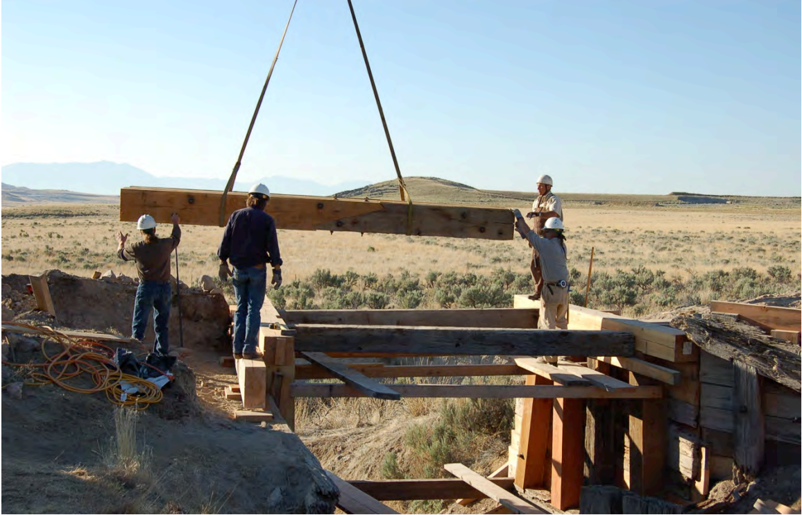
Figure 83: The crane lowers one of the completed stringer assemblies onto the trestle.
