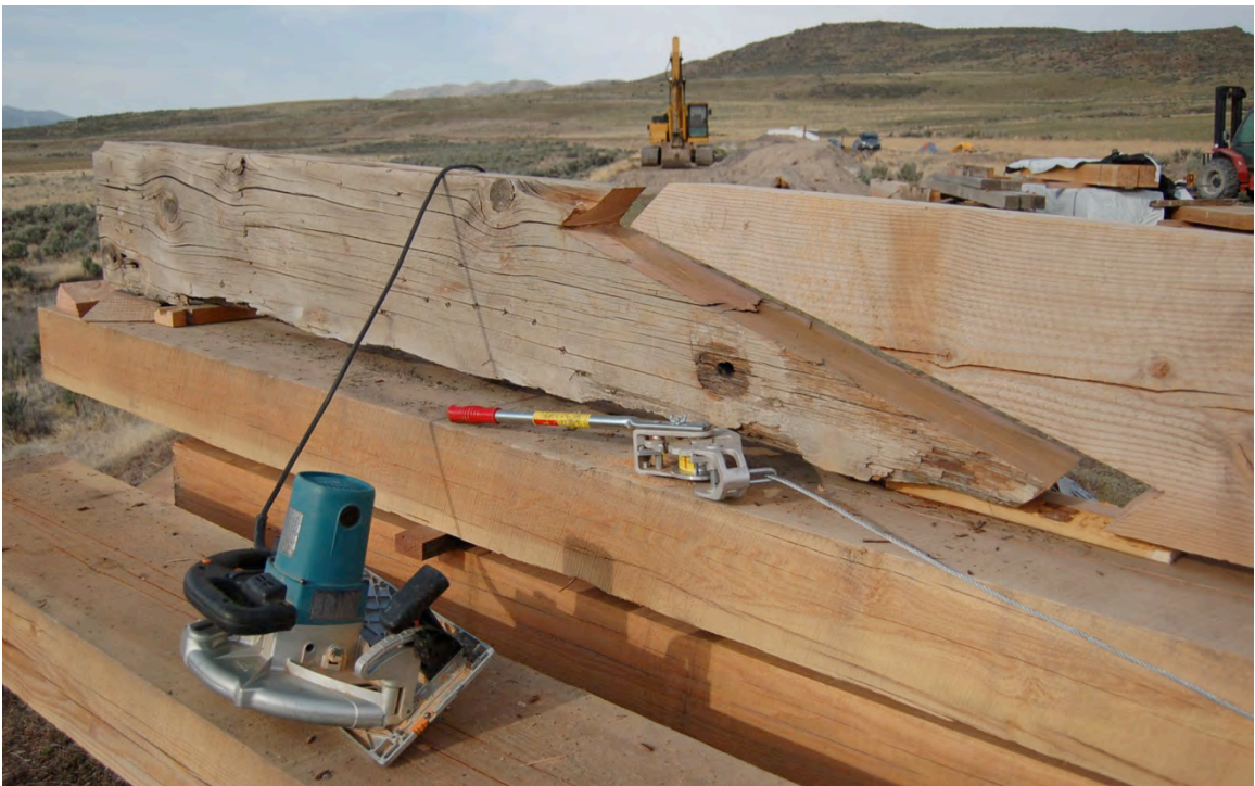
Figure 60: A scarf has been cut to repair one of the stringers of Trestle #1.
