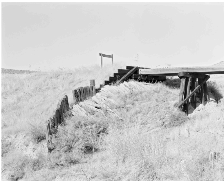
Figure 100: UT-64-4, Southwest view of trestle showing timber riprap installed by the National Park Service in the late 1970s.
