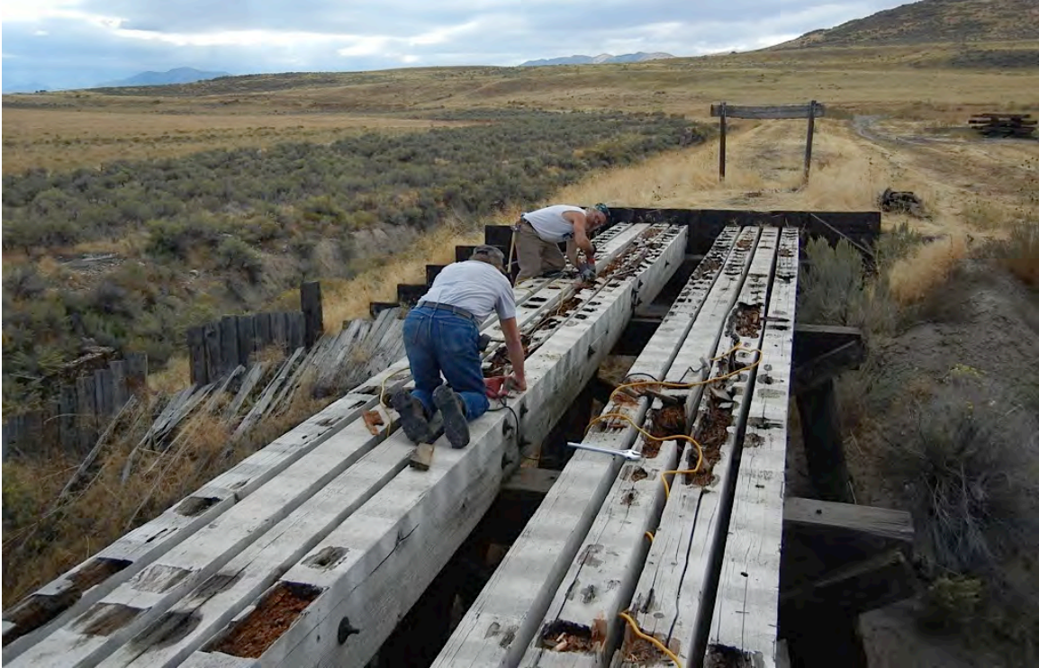
Figure 86: The stringers of Trestle #2 had significant pockets of decay along their length.
