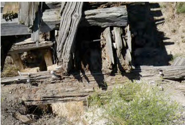
Figure 13: East pile cap (foreground) with severe deterioration.
