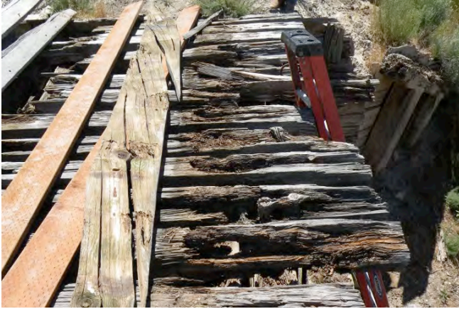
Figure 11: Deteriorated ties on Trestle #1.
