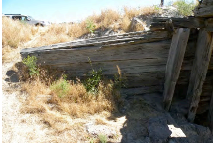
Figure 17: Northeast wing wall with surface and end deterioration.
