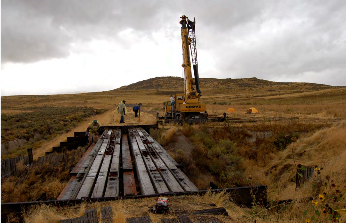
Figure 87: Planking was installed on either side and between the stringers assemblies to facilitate access and to act as guides for their eventual replacement.
