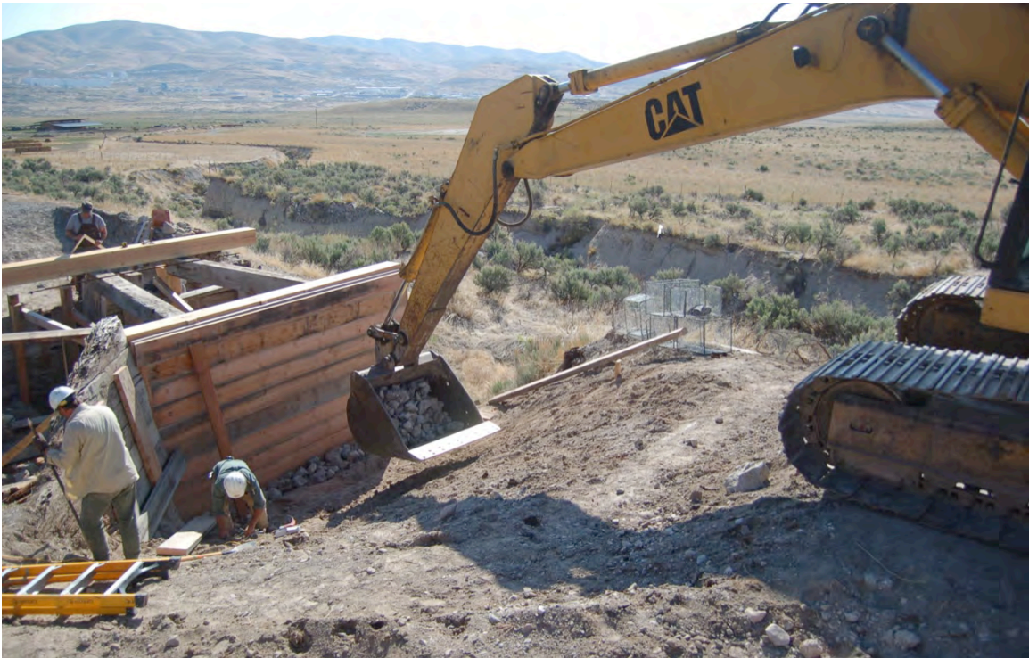
Figure 70: Large rocks were added behind the bottom of the west bulkhead to facilitate drainage.
