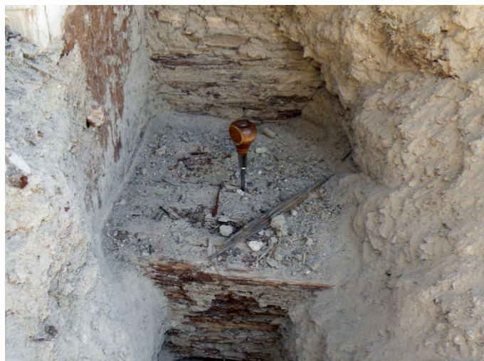
Figure 6: An awl can easily be inserted into the mudsill, east bent, Trestle #1.
