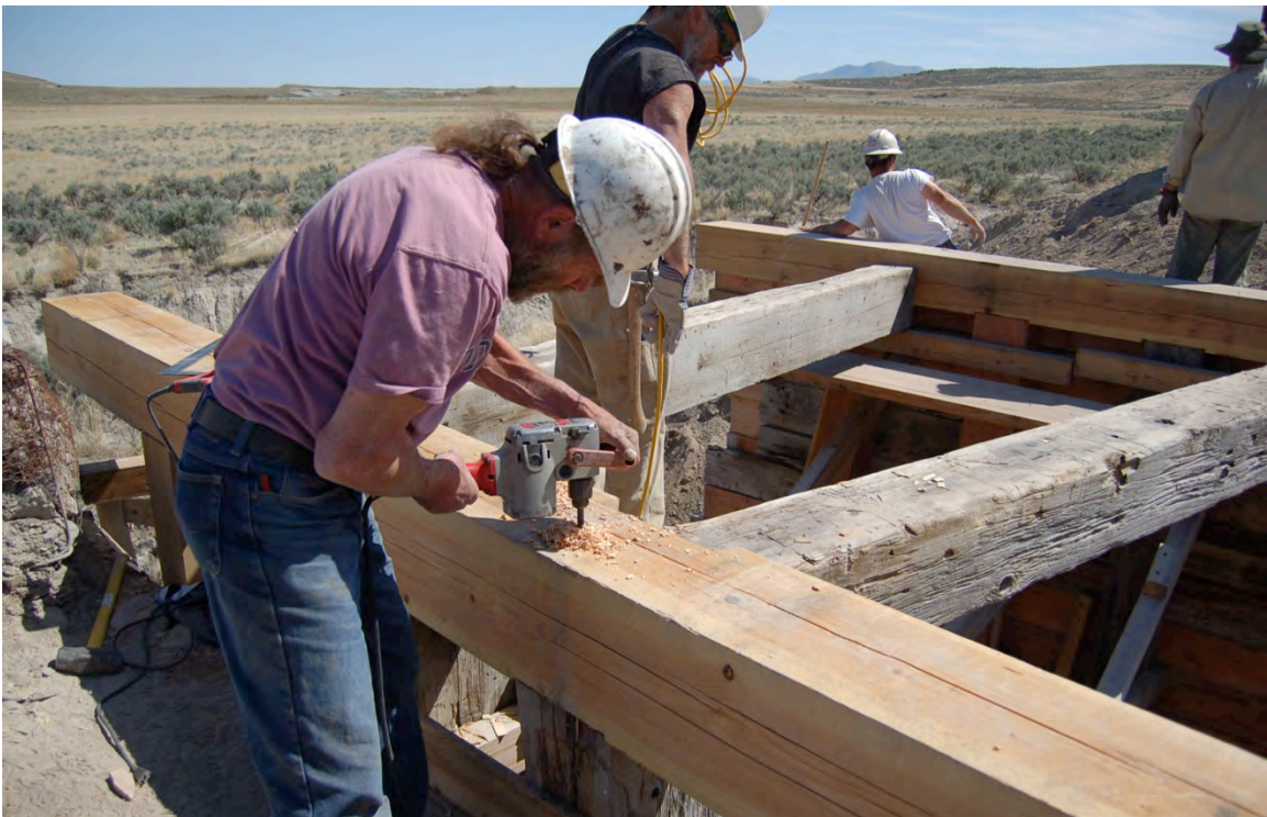
Figure 80: Drilling for hardware to secure the pile cap to the bent below.
