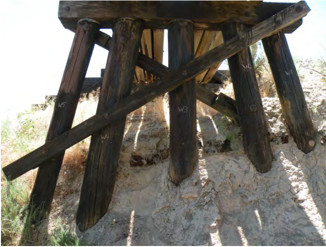
Figure 24: Creosote-treated west bent piles, Trestle #2.
