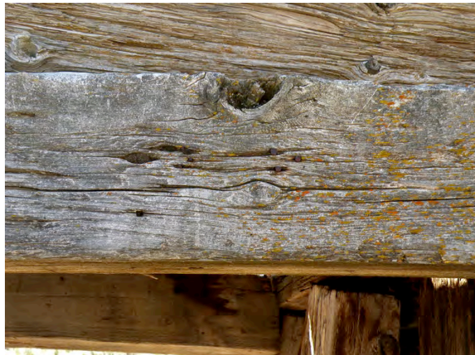
Figure 5: Example of an edge knot on the north strut of Trestle #1.
