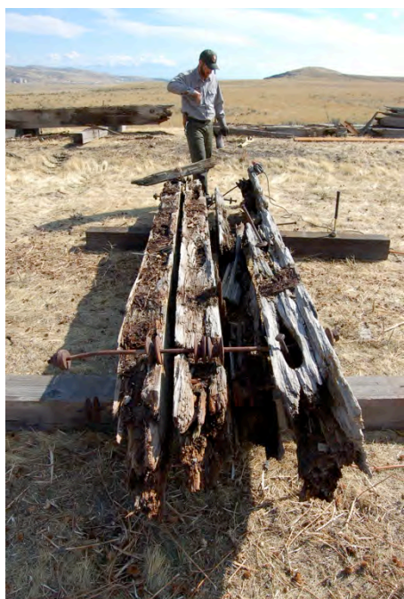
Figure 27: One of the original stringer assemblies removed from Trestle #1. Portions of two of the girders were salvaged and repaired for reinstallation.
