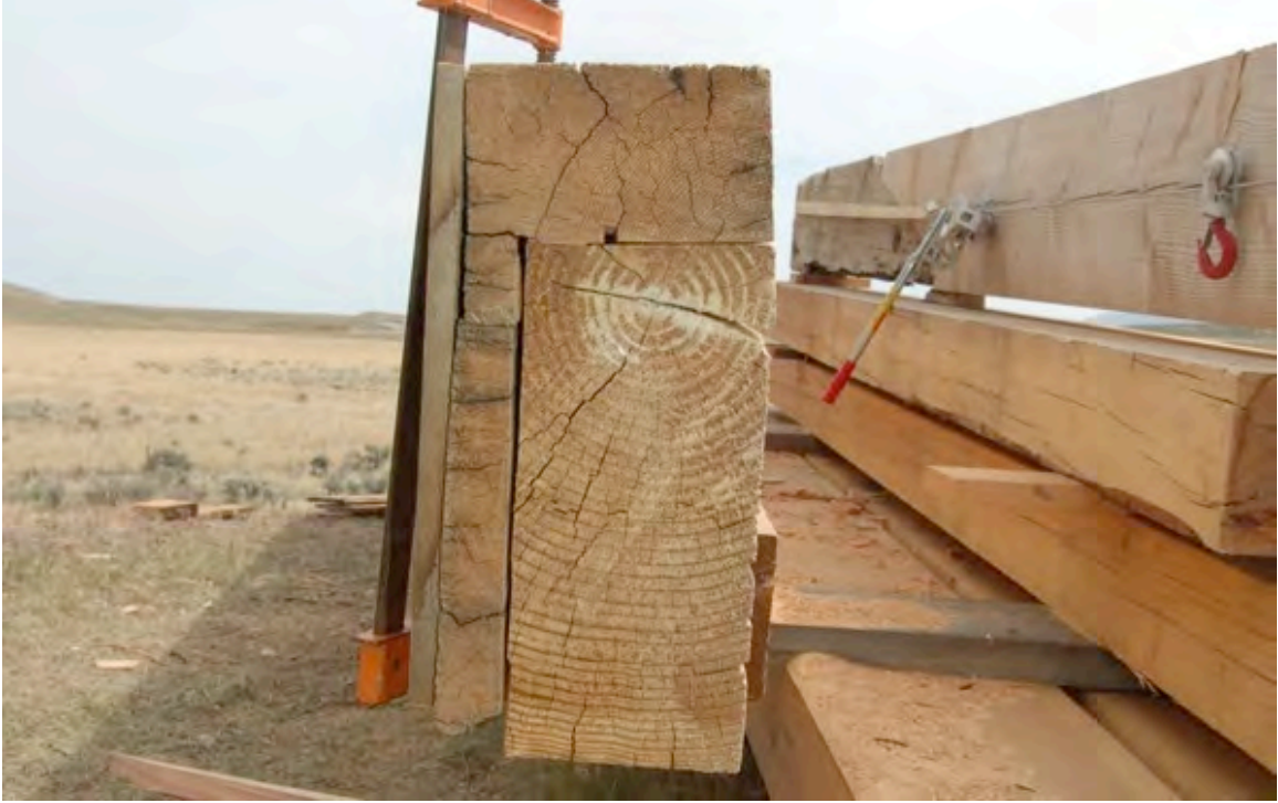
Figure 63: The repair for this stringer was a lap scarf that acts as a veneer over the new timber.
