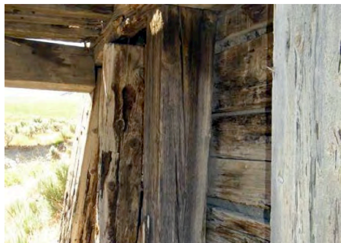
Figure 9: West bent of Trestle #1 showing slope of grain (W2, center) and large knots (W3, adjacent, left).
