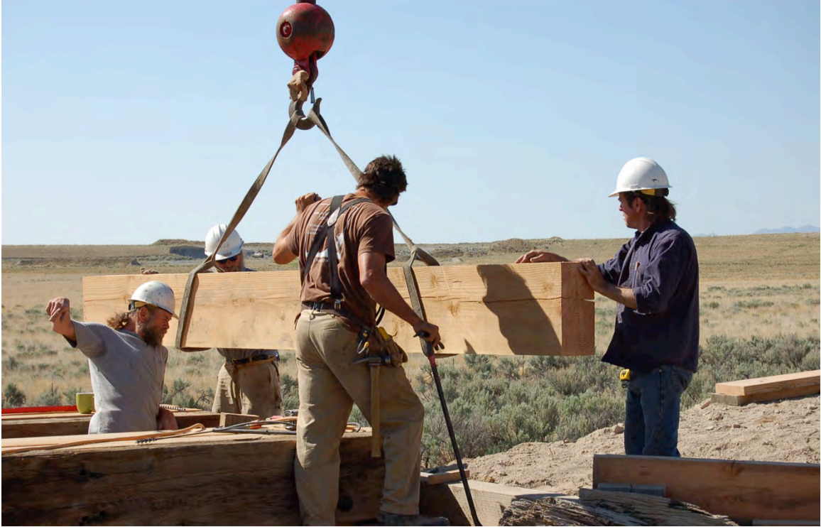
Figure 84: The last pieces to be installed are the top planks of the bulkheads.
