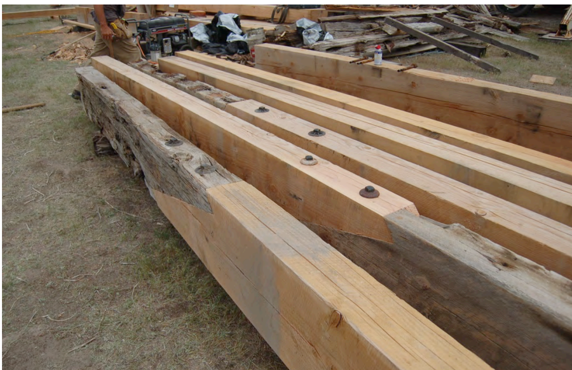
Figure 62: These scarf joints have been bolted together and the stringers are ready to be stacked into sets.
