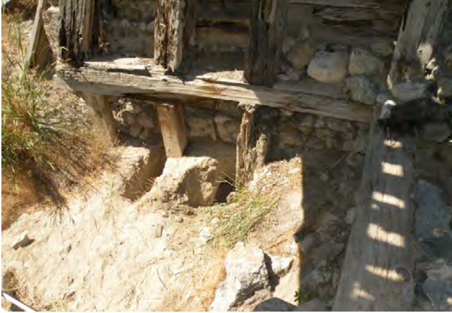
Figure 16: West bent intermediary sill with some decay. The two supporting piers to the left were replacements, and the older piers to the right were largely lost to decay.
