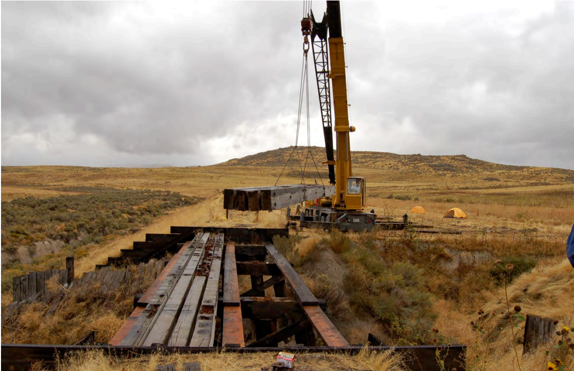
Figure 88: A crane was used to remove the assemblies from the trestle structure.
