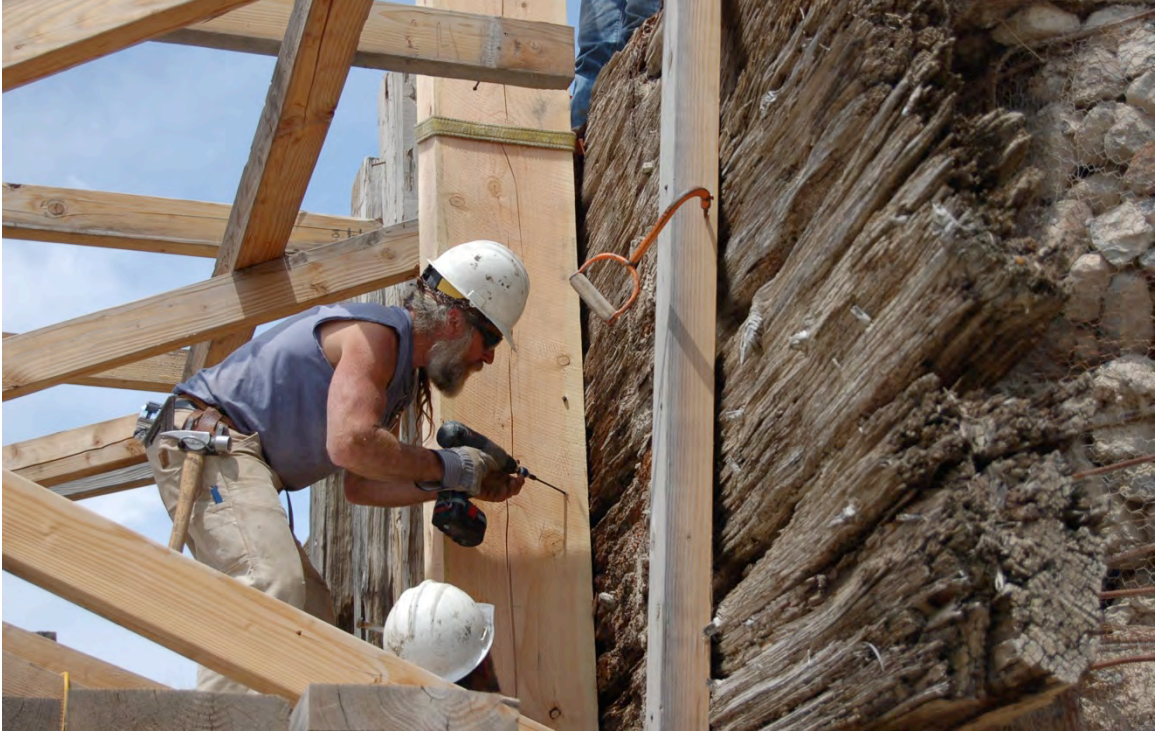
Figure 59: The replacement pile is tacked to the surrounding structure and then braced until a new pile cap is installed.
