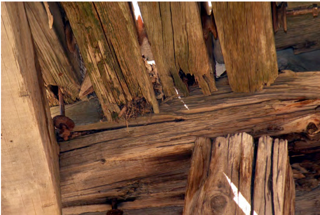
Figure 12: Deterioration at the bearing areas of the stringers.
